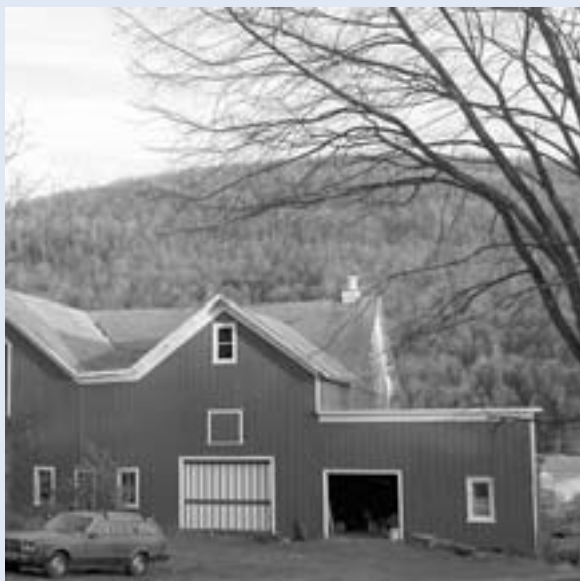
Richard Giles and Holley White completed barn repair, painting and landscaping to beautify their organic vegetable and retail farm on Route 10 in Hamden.
