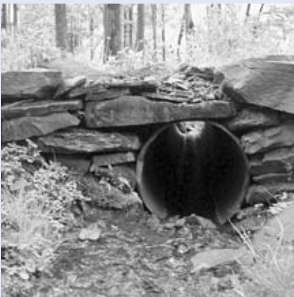
To date, loggers in the Watershed Forestry Program have stabilized over 478,096 linear feet of forest roads with BMPs, including the installation of over 1,820 erosion control culverts.
